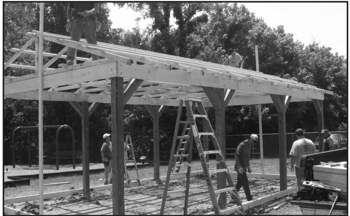
VOLUNTEERS FROM THE Parkersburg-Marietta Building Trades Council build a 16 by 30 foot covered shelter for their "business partner" the Fairplains Elementary School in Parkersburg.
