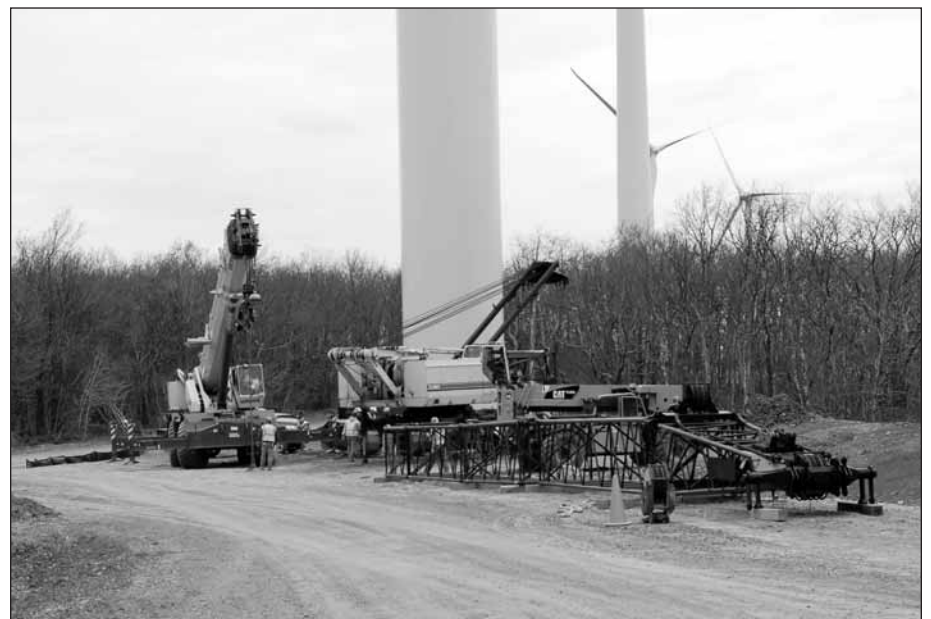
Union workers assemble a crane during the first phase of the Beech Ridge wind project in Greenbrier County. Only 67 turbines were erected out of the 122 planned. Soon another 33 turbines, at new locations, will be installed by local union construction workers.
