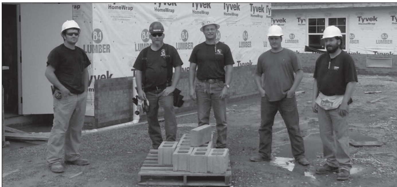
From left Ryan Melton, Jason Cobb, Dave Santrock, Tim Edens and John Null are five of the seven IBEW members working at the Devonshire project in Putnam County for LCN Electrical. LCN took the project over from nonunion Hi-Tech Electric in early June.
