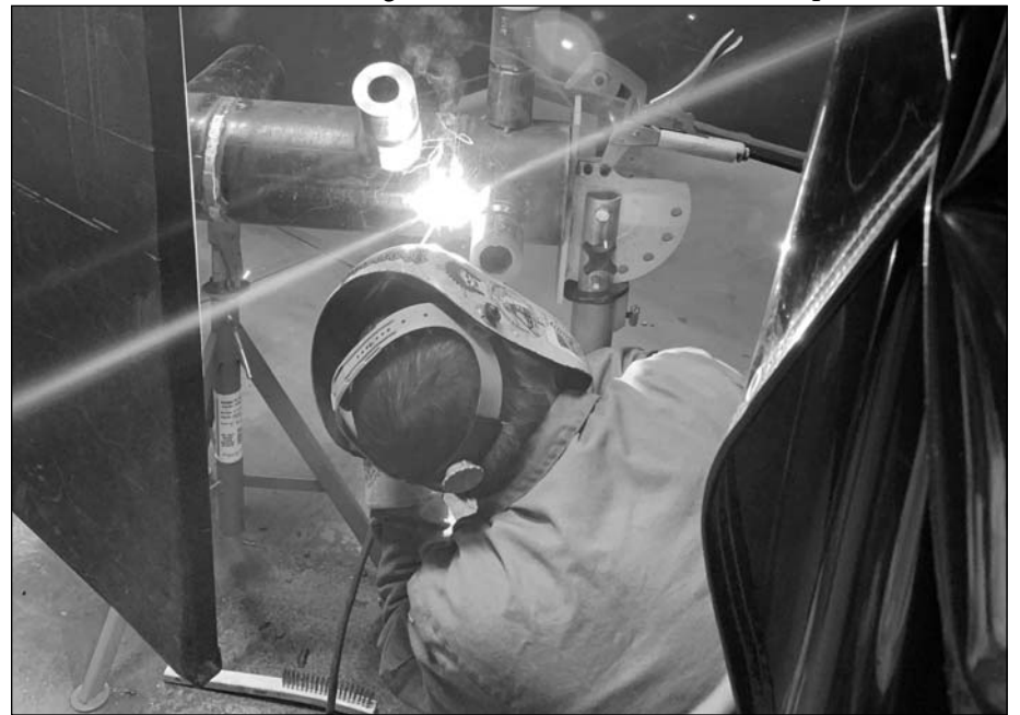
Andy Stanley from Morgantown Local 152 competes in the welding portion of the WV State Pipe Trades Apprenticeship Contest held in Charleston.
