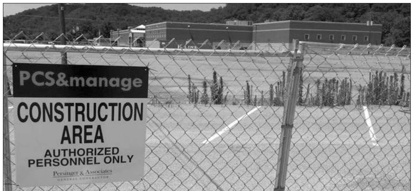
Construction of the Chapmanville Intermediate School started in spring of 2017 with a construction manager. Photo courtesy of Ryan Quinn, Charleston Gazette-Mail.
