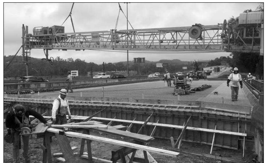
Union construction workers at the Danner Bridge portion of the Brayman Construction I-64 bridge re-decking project completed this section 24 days ahead of schedule.
