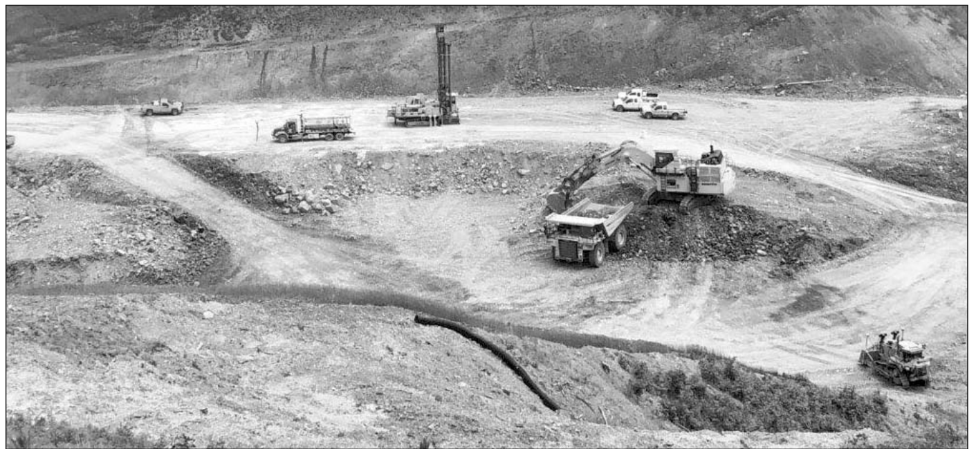
The night crew on this Corridor-H project was recently laid-off and more layoffs are expected due to permit delays. Kokosing is the general contractor on the Design-Build project.
