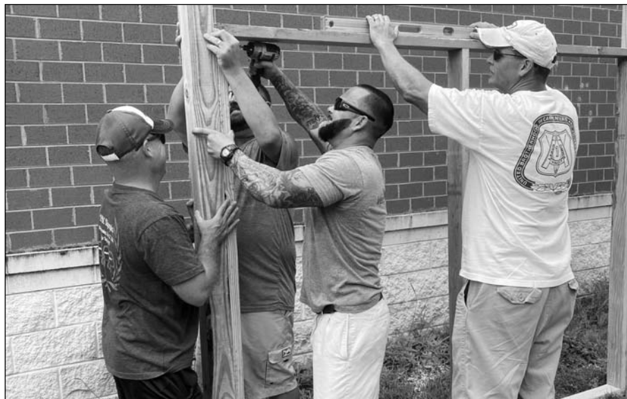
(From left) Randall May, Carpenters Local 439; Jeremy Jeffers, WV Training Director; Josh Nappi, Local 205; and Luke Begovich, Team Lead for the Eastern Atlantic States Regional Council of Carpenter, Charleston-Roanoke area, volunteer to build a K9 Obstacle Course in Roanoke, VA.
