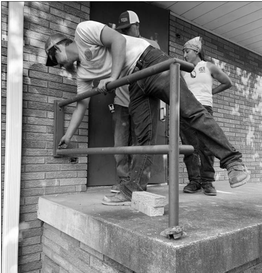
(From left) Iron Workers Local 549 Wheeling apprentice Dakota Wilson, Apprentice Instructor Todd Hebb and apprentice Nikke Renner volunteer at the Unity Center renovations in Benwood as part of the Project BEST commitment to rehab the facility.
