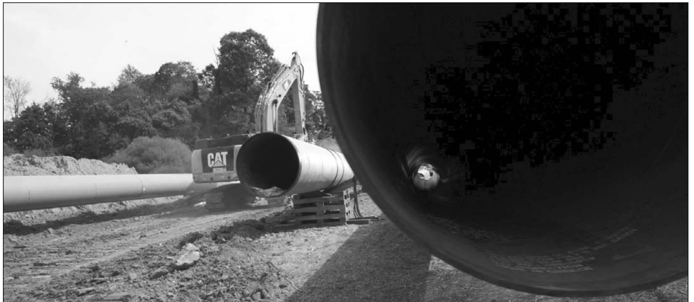
The Atlantic Coast Pipeline included 600 miles of pipe starting at Harrison County WV and ending in Virginia and North Carolina.
