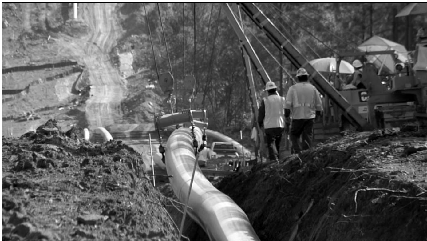
This pipeline construction picture comes from a promotional video for the ACP. The ACP has entered into a project labor agreement for the pipeline portion of the project and will use all union workers. For the compressor station and metering station work there is no agreement.
