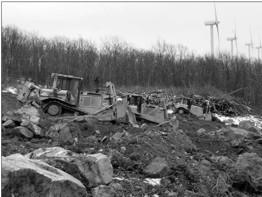
Operating Engineers Local 132 and Laborers Local 379 members are already working on site prep for the Black Rock Wind project in Grant and Mineral Counties. Other crafts should be on site starting in March.
